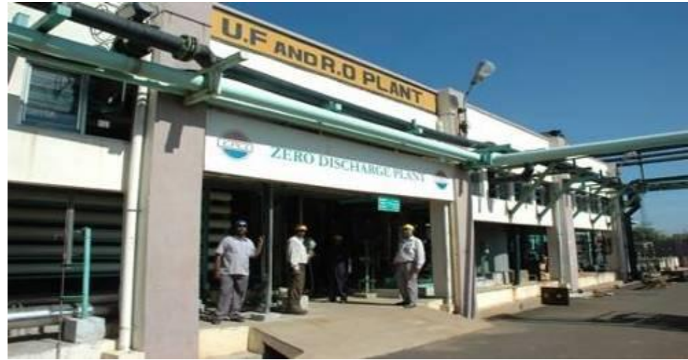
Zero liquid discharge set up at CPCL refinery Chennai
